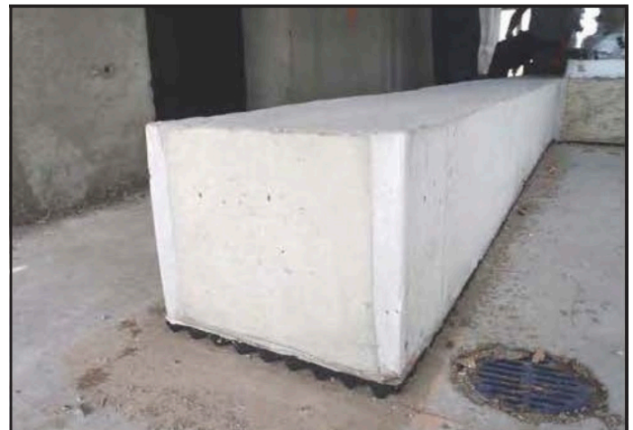
Properly isolated concrete pier for heavy equipment for example: chillers or cooling towers- ISO-SEP 25HD for lighter, and ISO-SEP- 25F for heavier applications.
